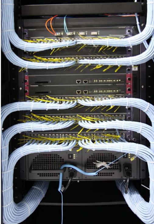
Figure 97 Network cable management
