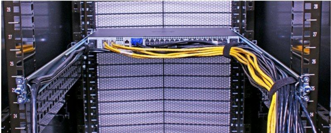
Figure 5: Four Post Rack: Routing Power and Data Cables
