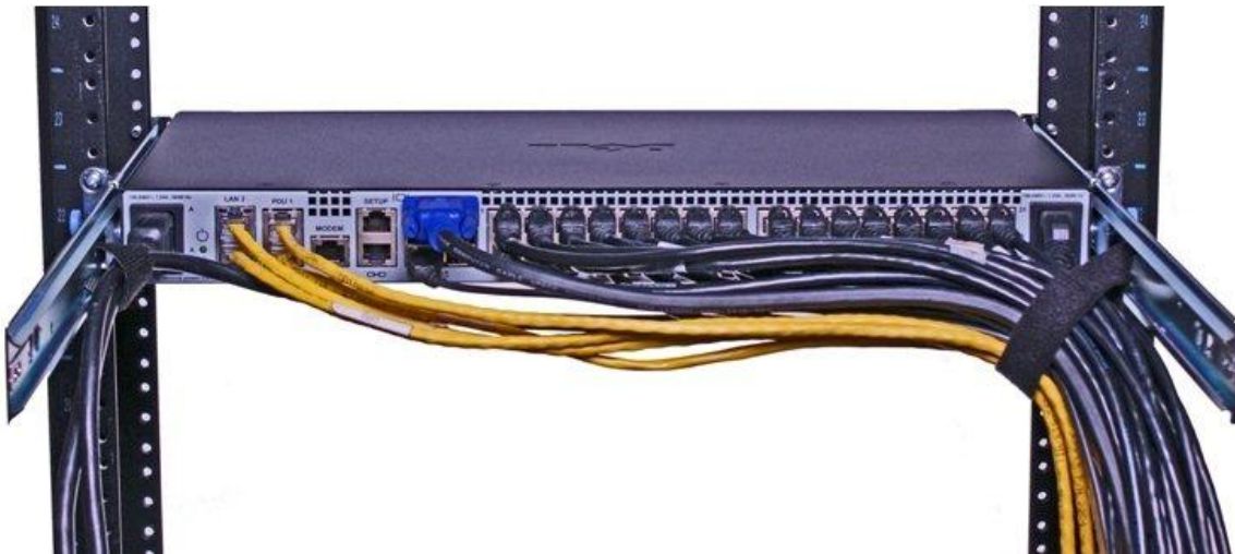
Figure 8: Two Post Rack: Routing Power and Data Cables
