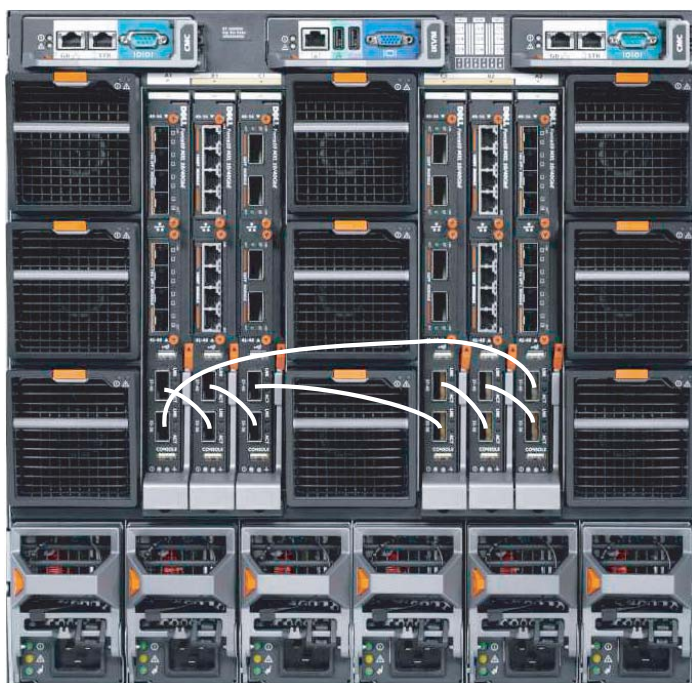
Figure 1-10. Six Stacked MXL 10/40GbE Switches
